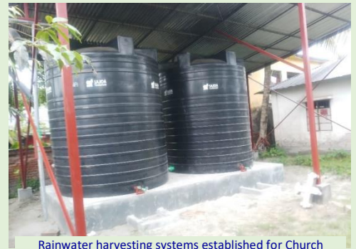
Rainwater harvesting systems established for Church through another NGO, the result of strong collaboration
