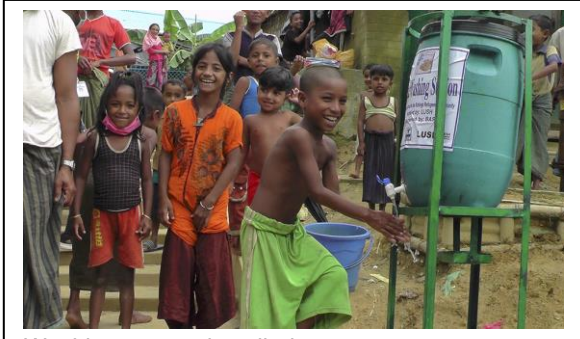
Washing system installed
